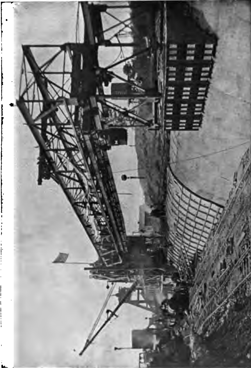
PLATE 71. —Contract 11. Traveling Crushing Concrete, Mixing, and Form-moving Plant Completing Last Section of Aqueduct Adjoining Shaft 1 of Contract 12. This plant built 7500 feet of aqueduct in two seasons.
